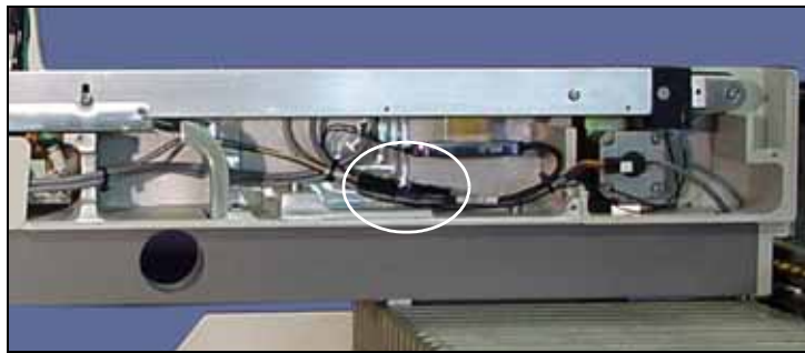
Figure P-21—Conveyor Wire Connector Locations (Circled)
