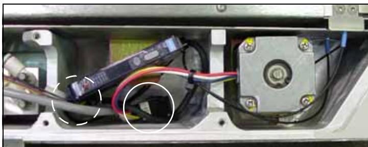
Figure F-21—Conveyor Wire Connector Locations (Circled) One is hidden by the cable. [MFU shown.]
