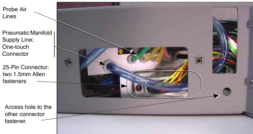
Figure F-16—Location of the Pneumatic Manifold Supply Line and Wiring Connector
