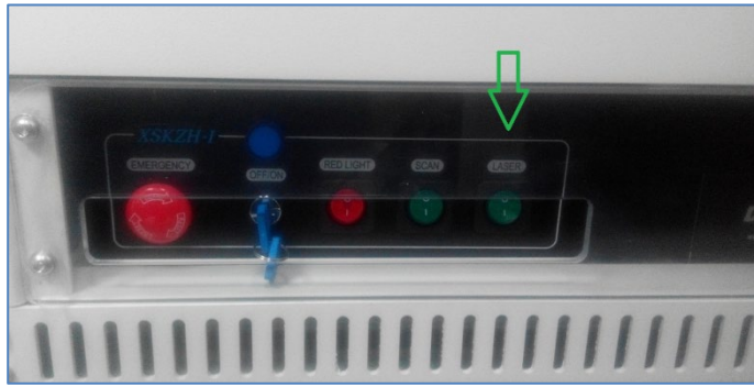
Figure 50: Laser Switch on the Laser power control panel.
