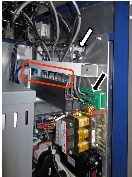
Figure 75: The right side connection panel inside the right front access door. Power cables (black arrow), Pneumatic manifold (white arrow),
