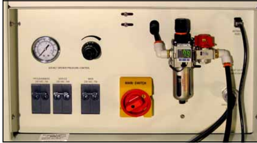
Figure 1-9: Power Panel on the back of the PS Machine.
